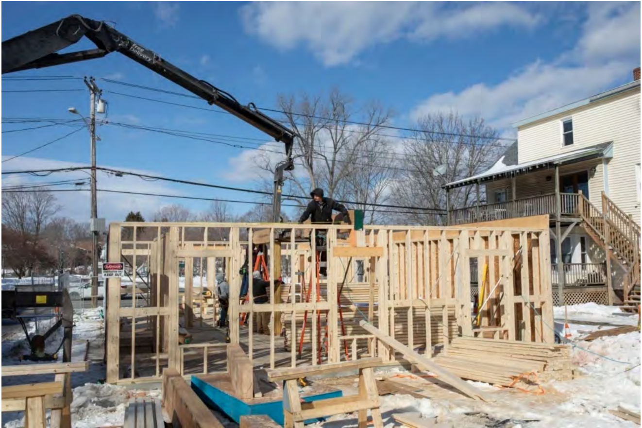
A crew works on framing the first floor of a multifamily building on Main Street in Westbrook on Feb. 11. Brianna Soukup/Staff Photographer
